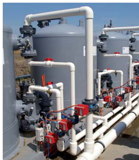
Resin bead filters initially reduce particles in the water down to 50 microns before the water is pumped into the RO unit
