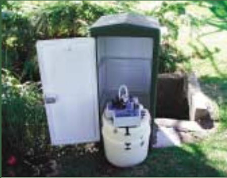
The stormwater sampler at Manly Golf Club
