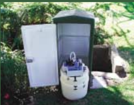
The stormwater sampler at Manly Golf Club
