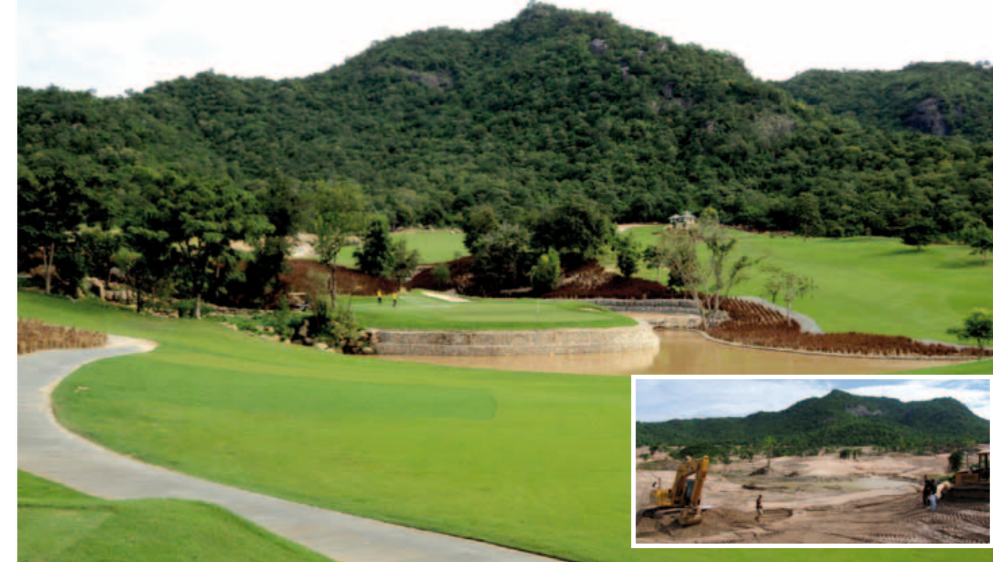
The Black Mountain Golf Course in Hua Hin, Thailand as it is today and (inset) as the site looked during construction in mid-2006
